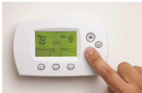
Figure 14: Room temperature control panel
